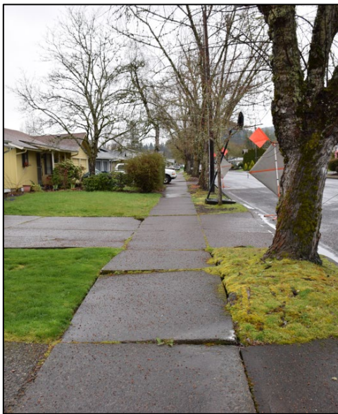
Sidewalk uplift will be repaired to make Springfield more accessible
