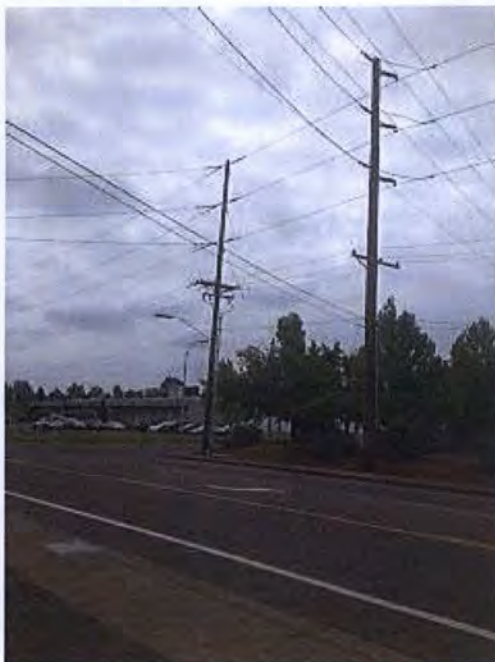
Transmission lines on Laura Street near the Laura Street Substation
