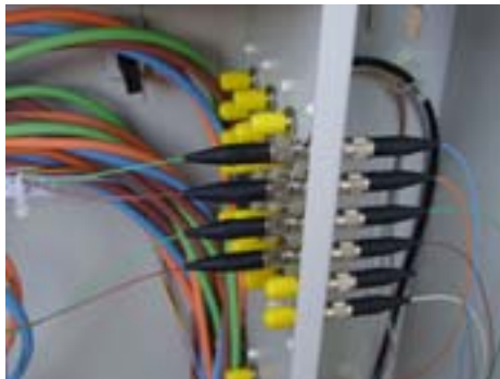
Fiber Optic Cable Terminations
