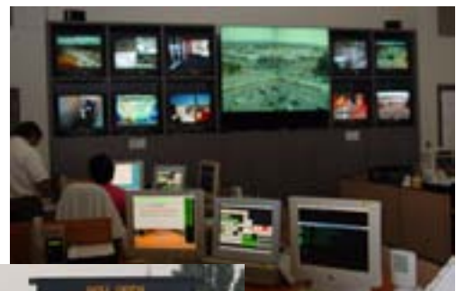
Northwest Transportation Operations Center (NWTOC)
